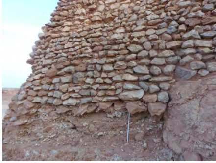
Fig.3- Aghem of Taguelzi. Constructive detail of the stone boundary walls (Illili Mahrour, 2015).
