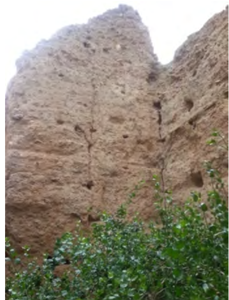
Fig. 5- State of degradation vertical cracks in walls (Abdessemed-Foufa, 2016).
