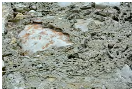
Fig. 7- Weathering of plaster.
